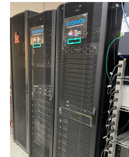
Servers hosting O-RAN end-to-end and automated data collection
